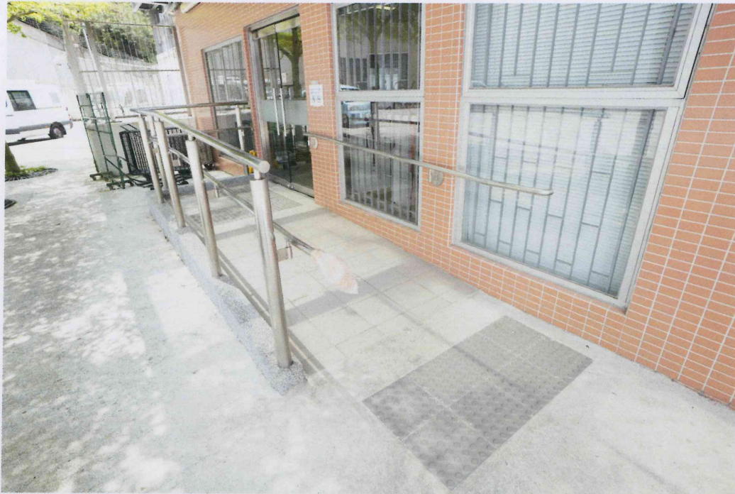
Barrier free ramps installed to connect the car parking space and the entrances at ground floor (G/F)
